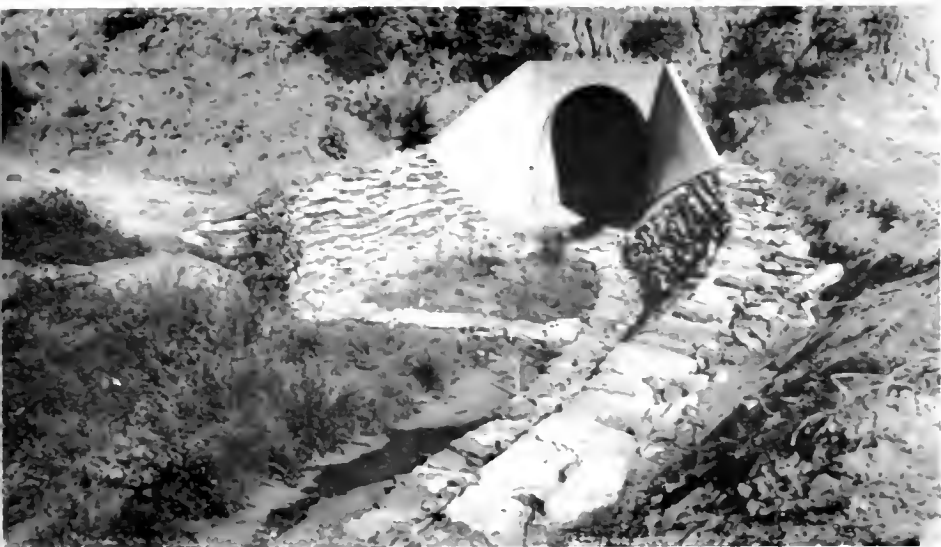
FIG. 37. Warped endwall proved too short. Transition extended by supplemental design
